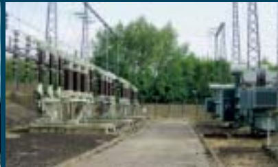
power distribution station
